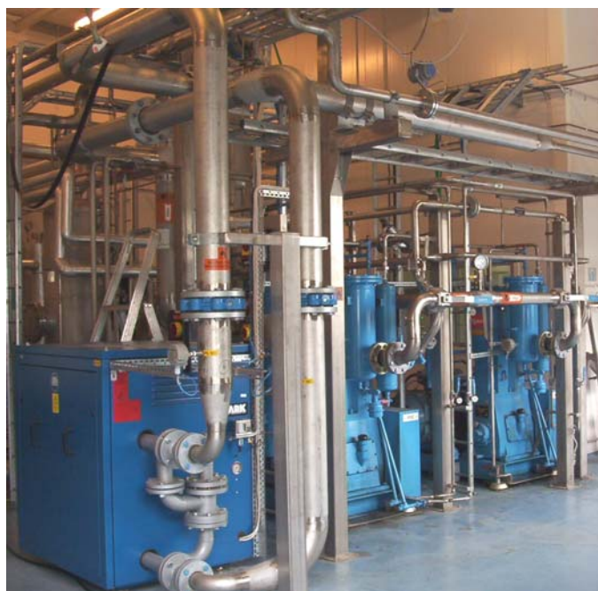
Water scrubber is the most common method to separate carbon dioxide. This plant is situated in the town of Kristianstad.
